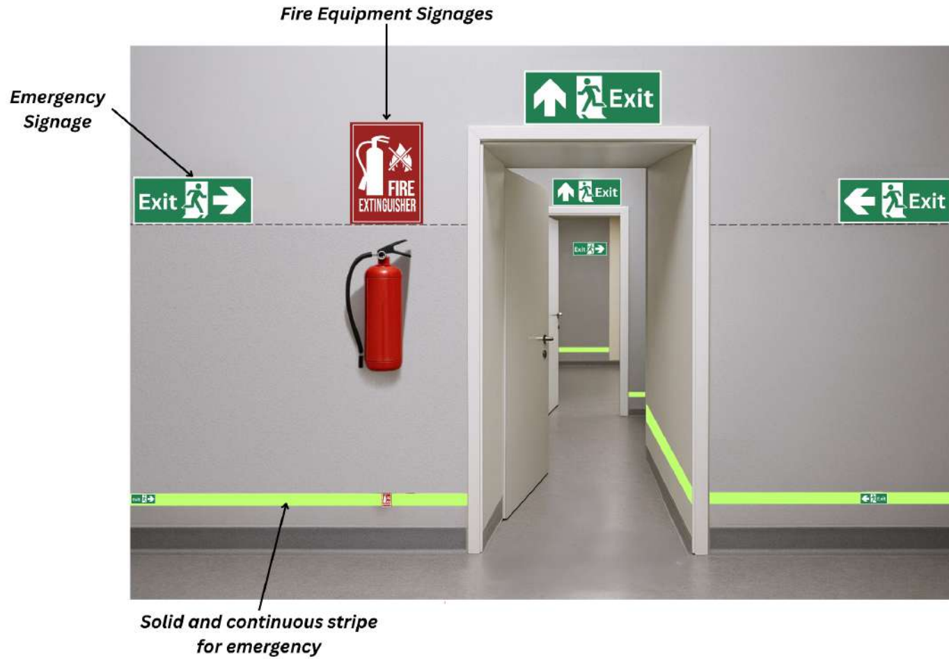
Figure 8: Example of Safety Signage
